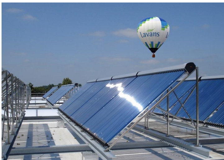
Solar heat collector on the roof of the Lavans laundry
